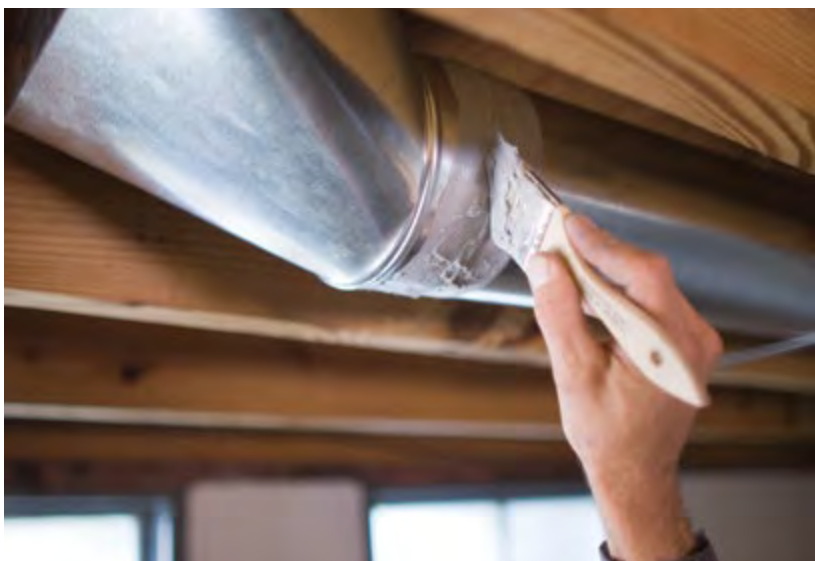
Sealing duct work in the home can help improve the overall efficiency of the air conditioner.
