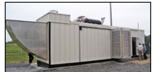
This 1,000 kW diesel generator is one of two generators recently installed by LJEC.
